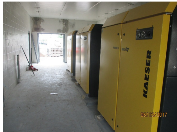
View of the 3 blower units placed on the concrete equipment pads within the Blower Room area.
