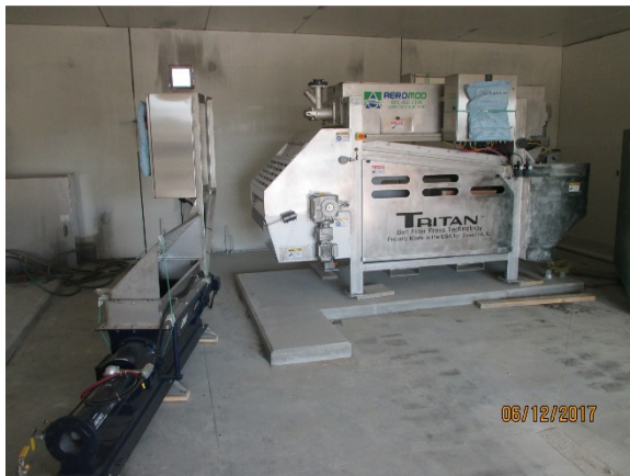
View of the sludge cake pump and the sludge press within the Sludge Press Room area.
