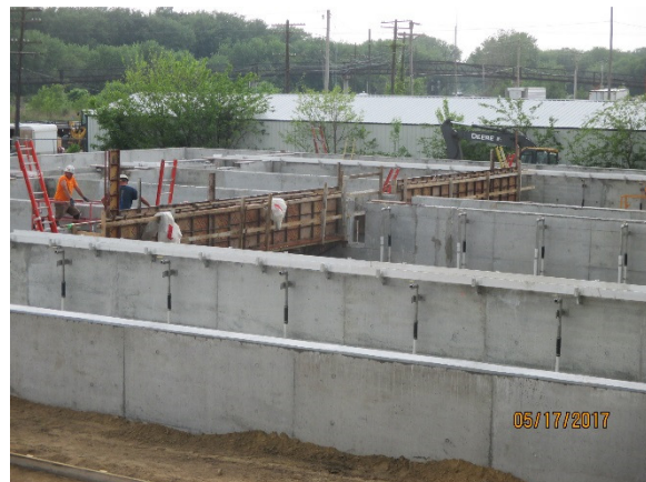
Placing concrete at the RAS Trough section of the Aeration Tanks at the Aero-Mod tank.
