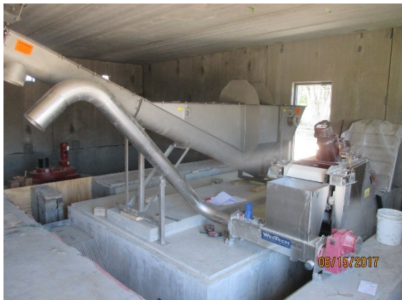
View of the grit classifier and stair screen positioned within the Headwork's Room area.
