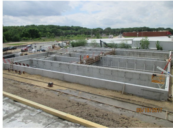
Overall view of the completed Aero-Mod tank and completed aeration piping and valves
