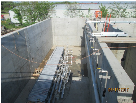
View of the installed aeration piping and ball valves at the Digester Tank section of the Aero-Mod tank
