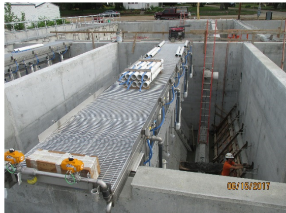
View of the Clarifier walkway with air fittings supplied by Aero-Mod.
