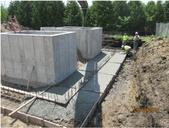
View of the placed concrete and steel reinforcement for the outer structure of the Main Street lift station
