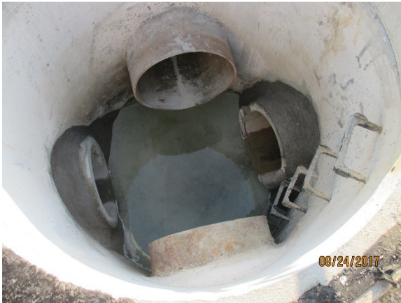
24" RCP outfall sewer and 30" cast iron storm sewer. Crossing at M.H. 6-B.
