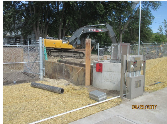
Excavating at the site lift station for the tie-in of the 8" PVC gravity sewer along Oak Street.
